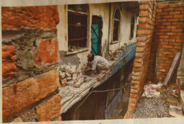
Reconstruction work in progress at Madeena Masjid in north-east Delhi's Shiv Vihar. © SHIV KUMAR PUSHPAKAR
